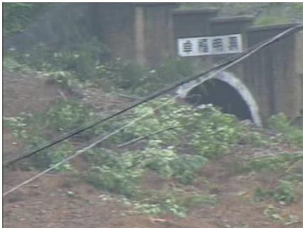
图 5 泥石流淤埋的卓福隧道 Fig.5 Zhuofu tunnel buried by debris flow
